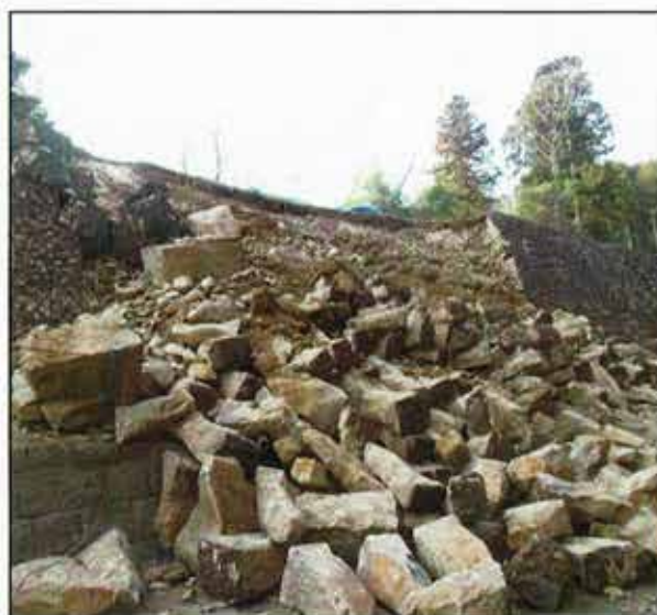
①石垣崩落
